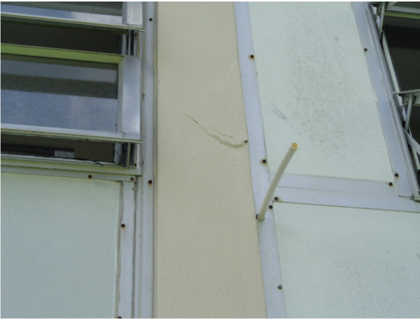
NCI-3: Column spalling between unit 157 &158
