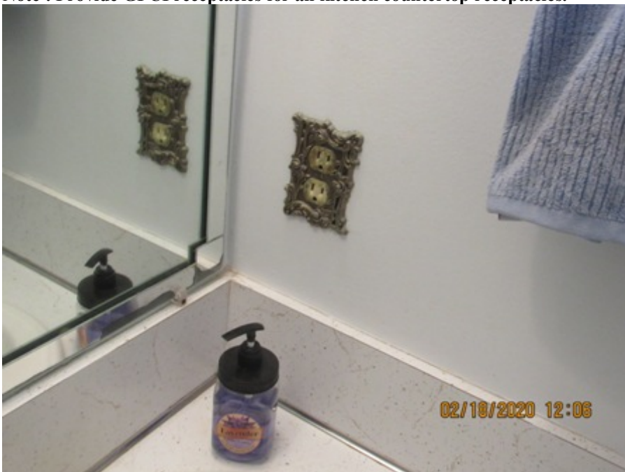
Photo 12: Apartment bathroom (Typ of 20).
