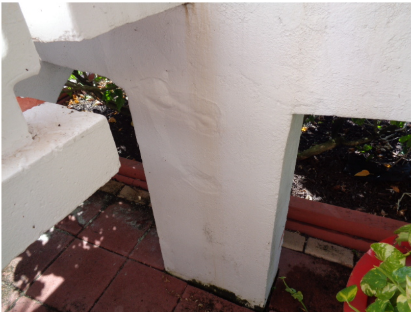
NCI-2: Column spalling at SE stairways
