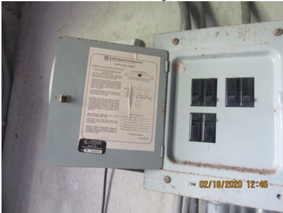
Photo 1: Main electrical room- House panel I
