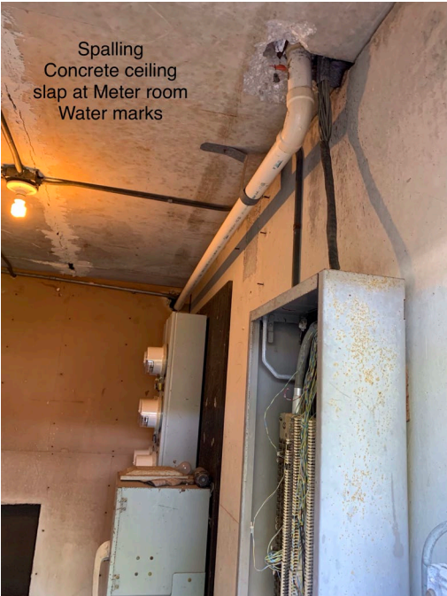
NCI-4: Spalling in concrete ceiling slab Meter room
