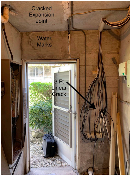
NCI-5: 3 FT linear wide crack, misaligned door frame and water marks in meter room
