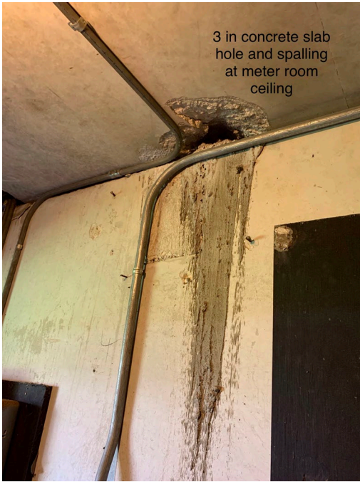
NCI-7: Third spalling concrete ceiling slab in meter room
