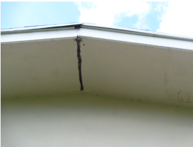
Figure 2..Open miter joints at ridge and fascia
