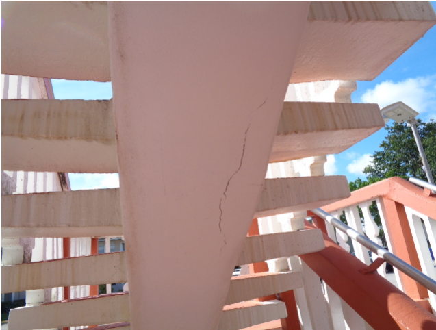
Figure 9...West stair beam spalling
