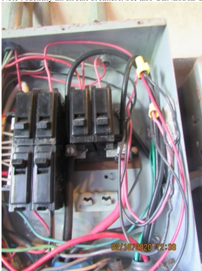
Photo 2: Main electrical room- House panel I
