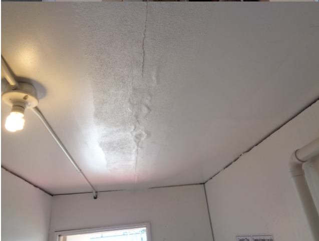
Figure 8...Expansion joint at laundry room shows spalling in joint proximity
