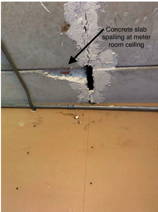
NCI-6: Second spalling concrete ceiling slab in meter room
