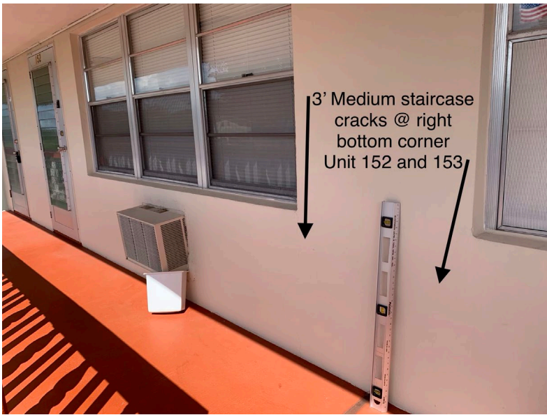
NCI-8: (2) Two 3 Ft medium staircase bottom window corners
