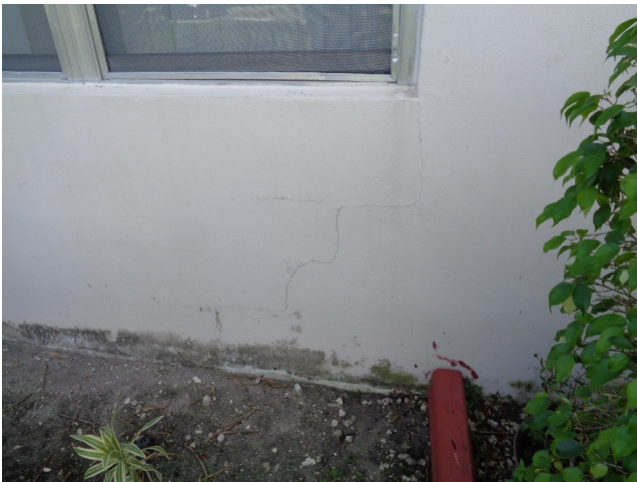
Figure 10...Stair case type cracking on wall west side.
