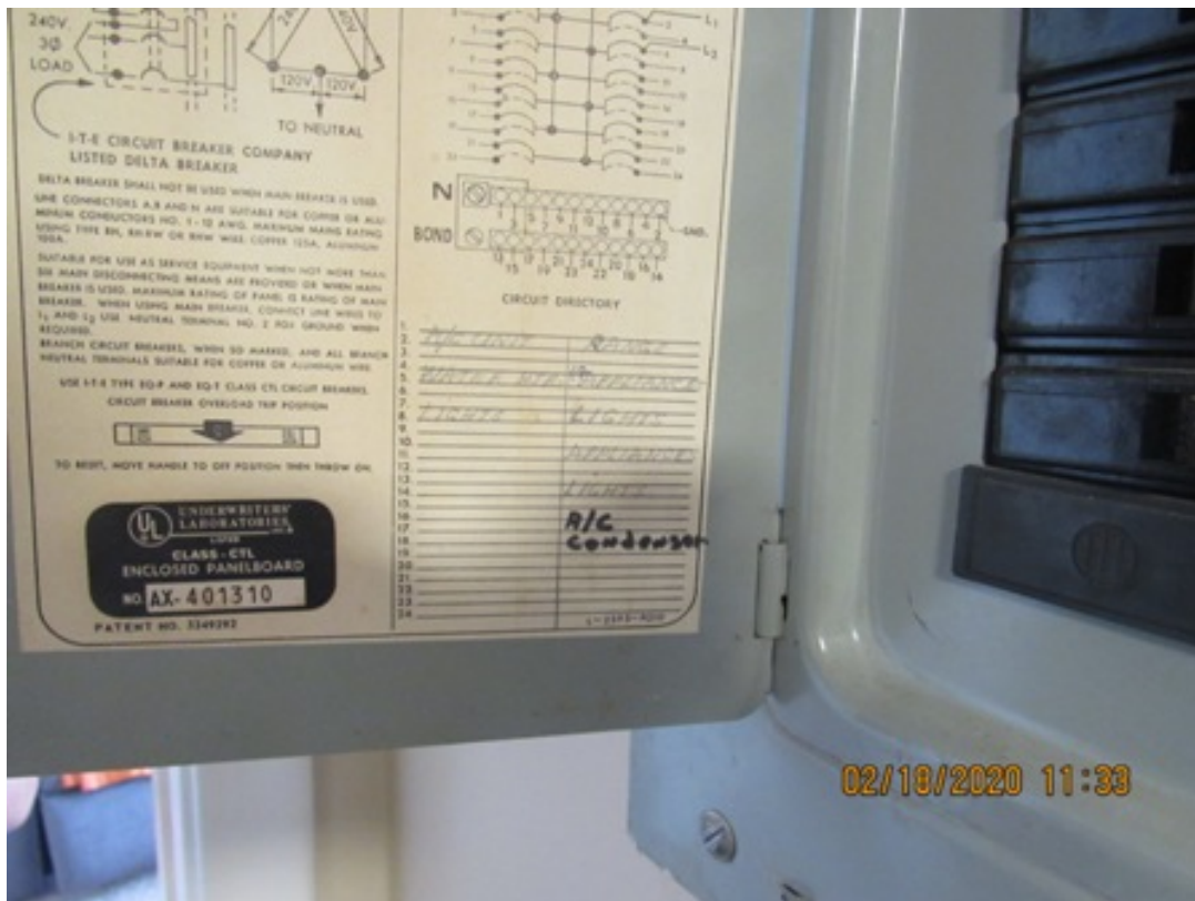
Photo 10: Apartment electrical panel (Typ of 20). Note : Identify all circuit breakers. See also GENERAL COMMENTS 2.0 on page 8.
