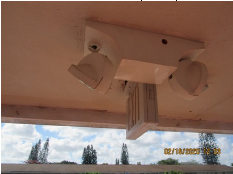
Photo 8 : Emergency /exit light combo
