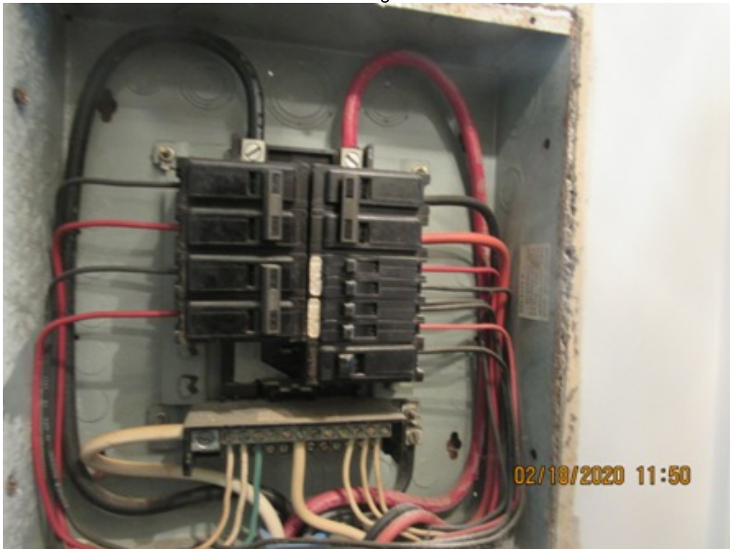
Photo 9: Apartment electrical panel (Typ of 20). Note : Equipment conductor shall be run with circuit conductors.
