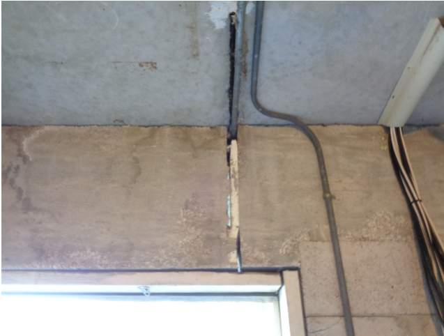
Figure 11...laundry room door should be sealed and finished, Also leaking expansion joint.
