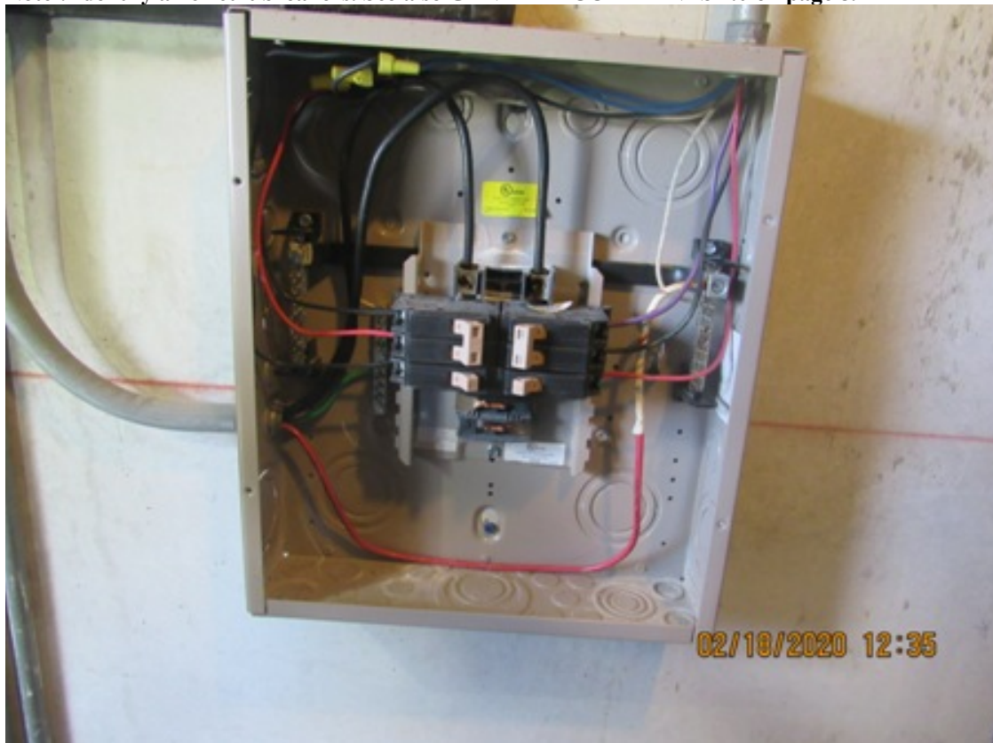
Photo 4: Main electrical room- House panel II
