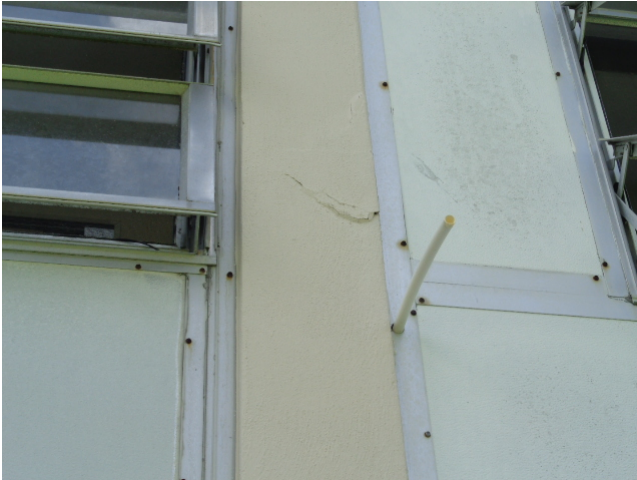
Figure 3...Column spalling # 159 Northside
