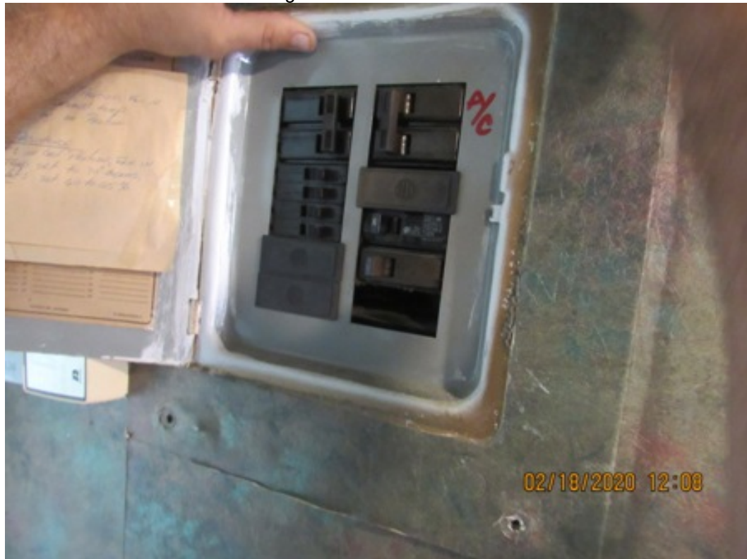
Photo 10: Apartment electrical panel #149
