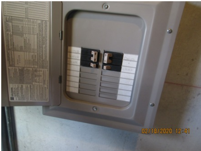
Photo 3: Main electrical room- House panel II
